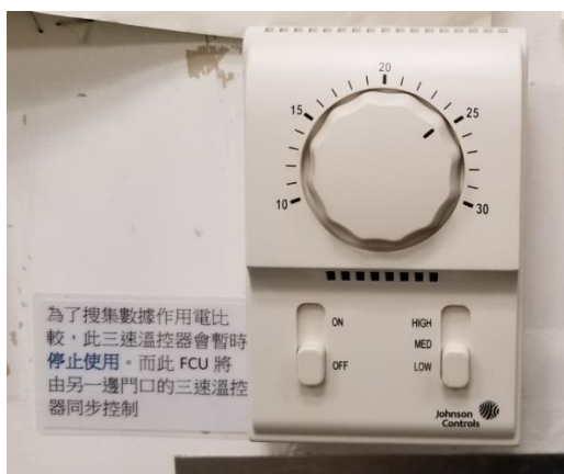
Photo 6 – 3-speed thermostat controller for the two FCUs
