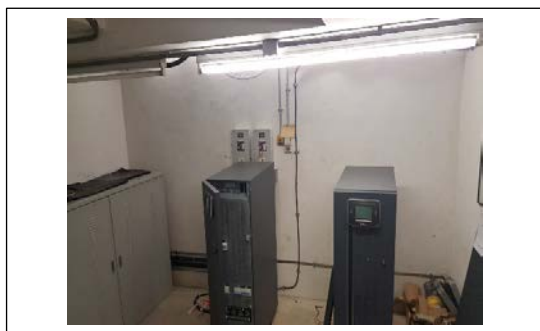
Photo 3. Old 40 kVA Reillo UPS
